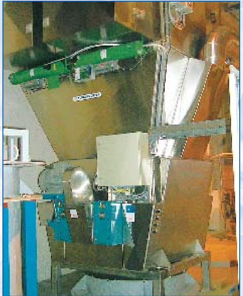
Forberg Mixer/Dryer FT-500 installed
